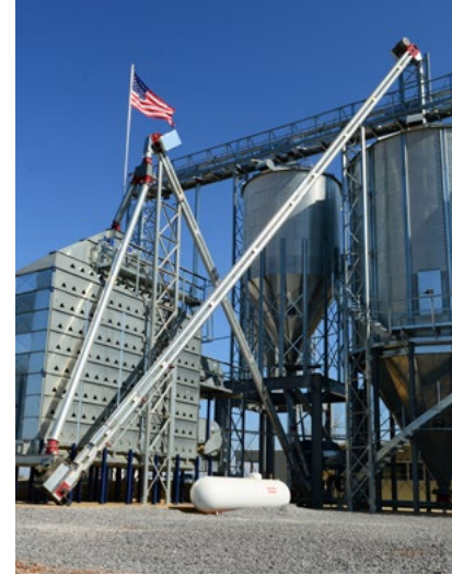
Stationary Double Run filling a dryer and unloading dryer to multiple bins.
